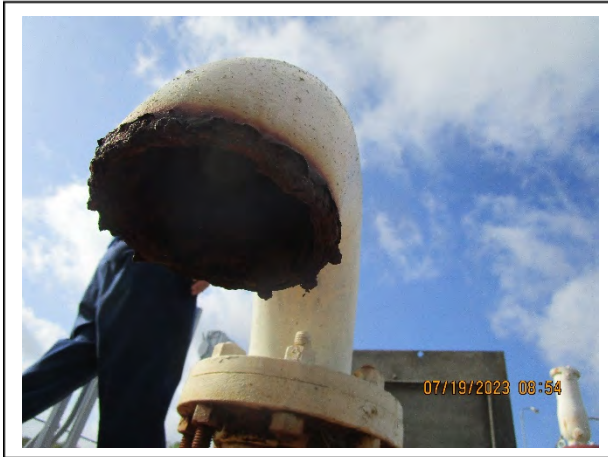
Findings: The wet well vent is corroded.
