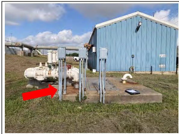
Findings: All three lift pump junction box supports are corroded. The conduit for the junction boxes are unsupported.
