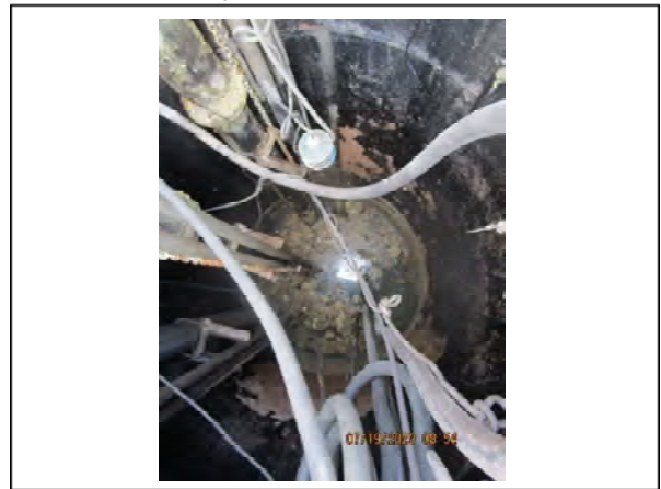
Findings: The lift pump electrical cables are not vertically supported.
